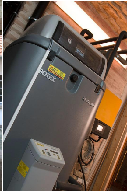
Hot water tank
