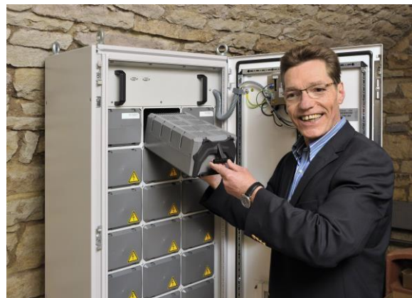
Lithium-ion battery for storing energy
