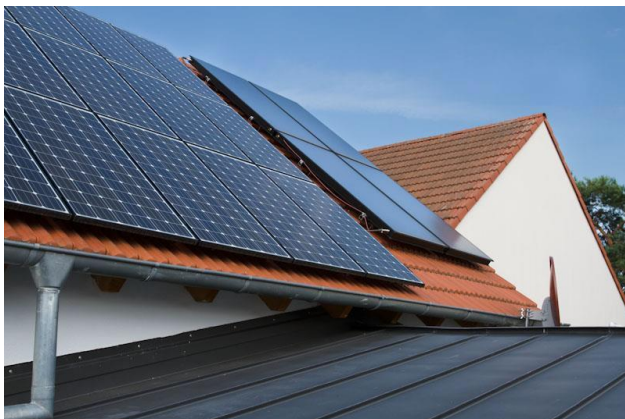
PV and solar thermal panels
