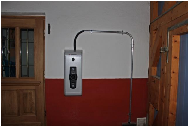
Solar recharging station
