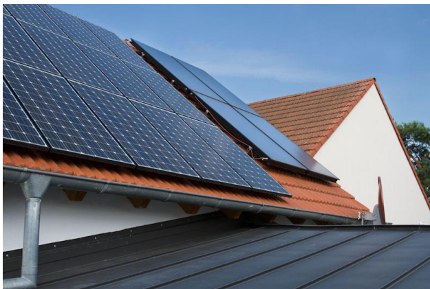
PV and solar thermal panels
